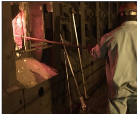
Ceramic welding end flue damage
