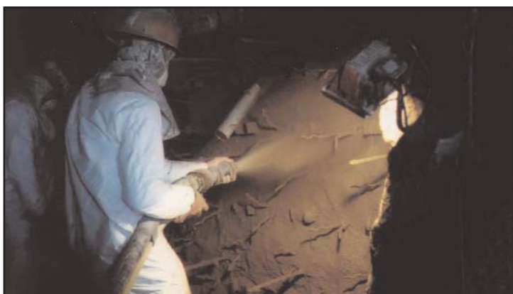
QUIKTURN™ 60G was a good selection for the firing hood lining at this Lehigh Valley cement plant.
