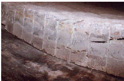
Figure one: Ring of brick adjacent to a fallen lining. Note the propagation of cracking from the cold end out to the hot face.
