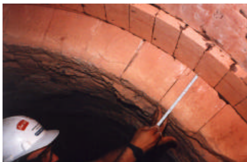
Figure five: Expansive alkali cracking in high alumina brick. Note the corners have cracked to relieve the pressure.
