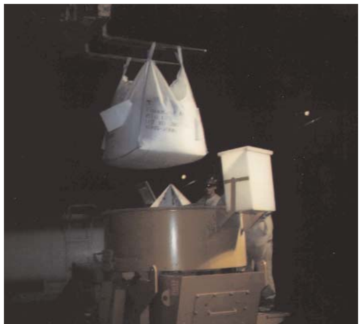
Control of the conditions during mixing affects the quality of a castable installation. It is especially critical to large pours.
