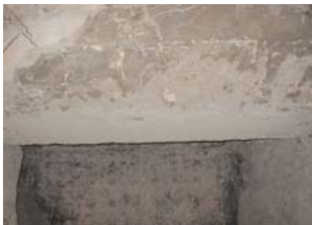
Figure 3. After one year of service, QUIKTURN 60PC remains a solid, durable refractory in this cooler bull nose.
