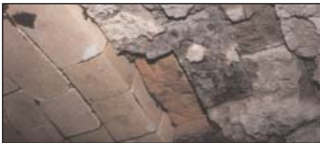
Figure 2. Alkali spalling in an insulated high alumina brick lining.
